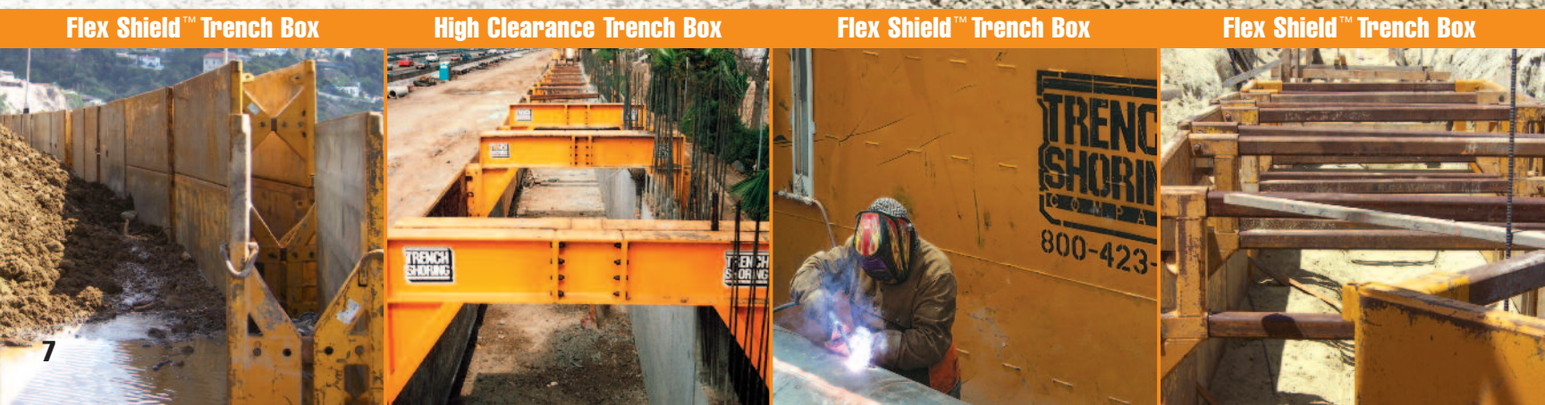
Poured in place box culvert 12'wide x 6'tall ID using 20' wide x 10' tall trench boxes end to end on the edge of Hwy. 118 Moorpark, CA
