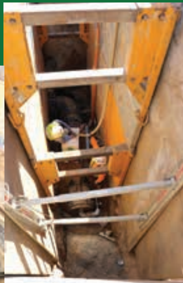
Above: 24" pipe in fire water trench.
