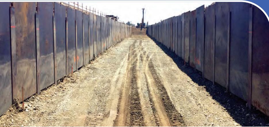
Below: West Fontana channel project sequence of operation. Trench Shoring Company provided hundreds of 8X15R Steel Plates to Sukut Construction on the project.
