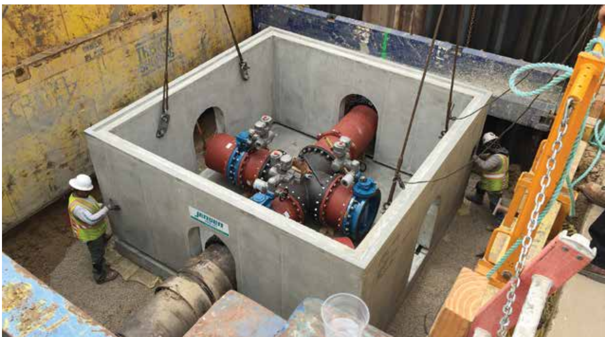
Trench Shoring Company’s Greg Shreenan credits an area’s “culture of safety” in helping to curb trench related incidents.
