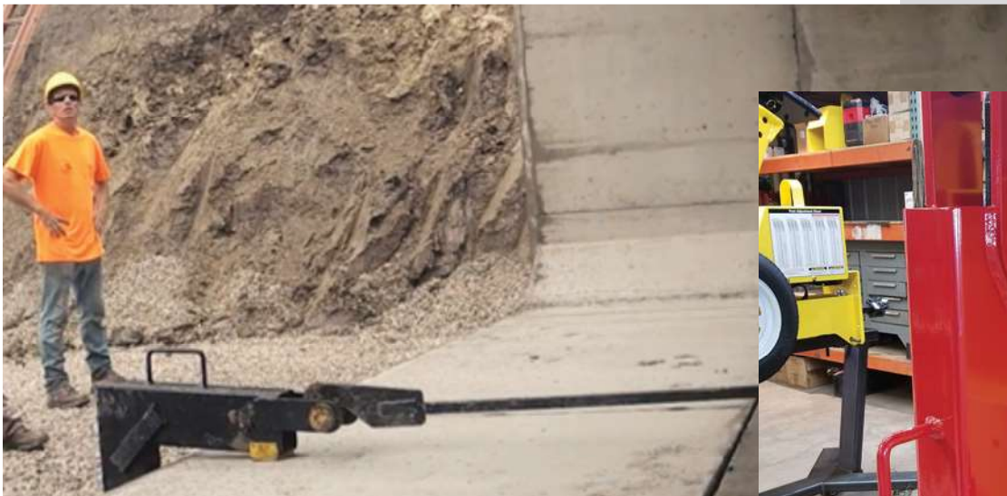
A J-Hook mounted on the side of a culvert.
